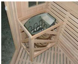
FIG-17 location of the stove
